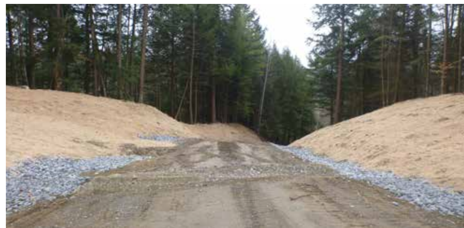
Steep section of truck road with stone lined ditches to prevent erosion. Also, good surface material helps maintain a good crown.
