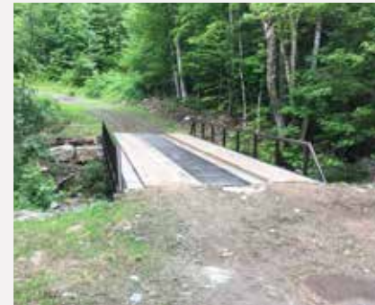
Temporary Truck Bridge
