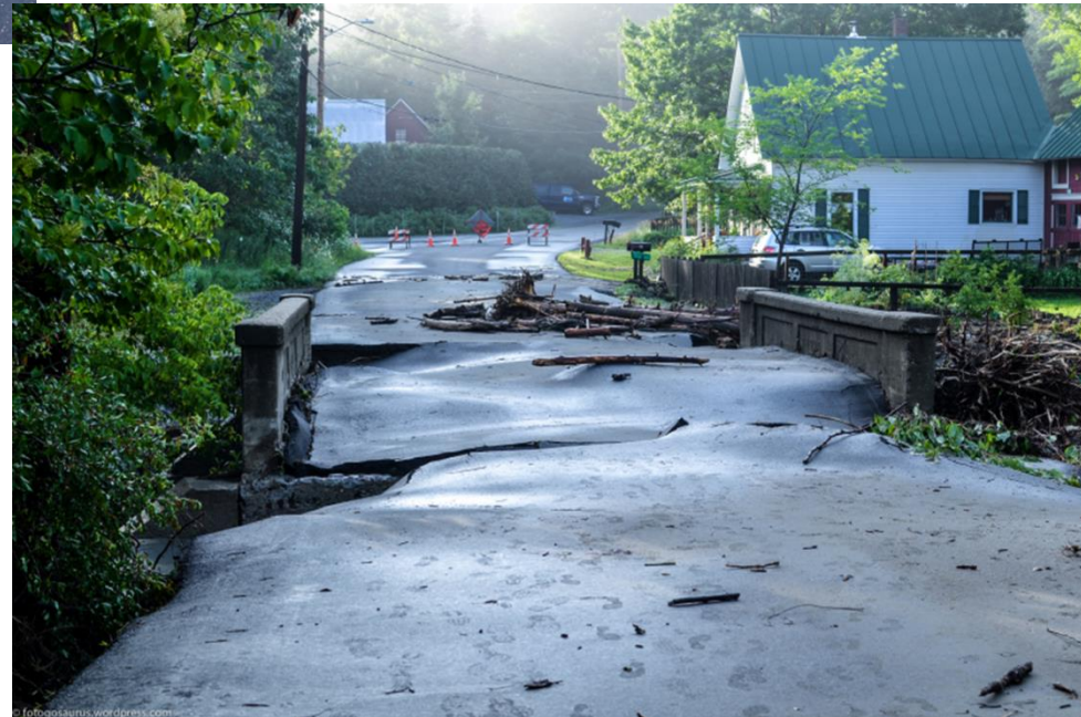
Great Brook Brook Road Damage, 10-Year Flood Plainfield, VT 7/20/2015 Photo taken by B. Towbin
