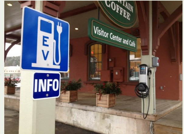
Waterbury EV Charging Station Photo: Brian Woods
