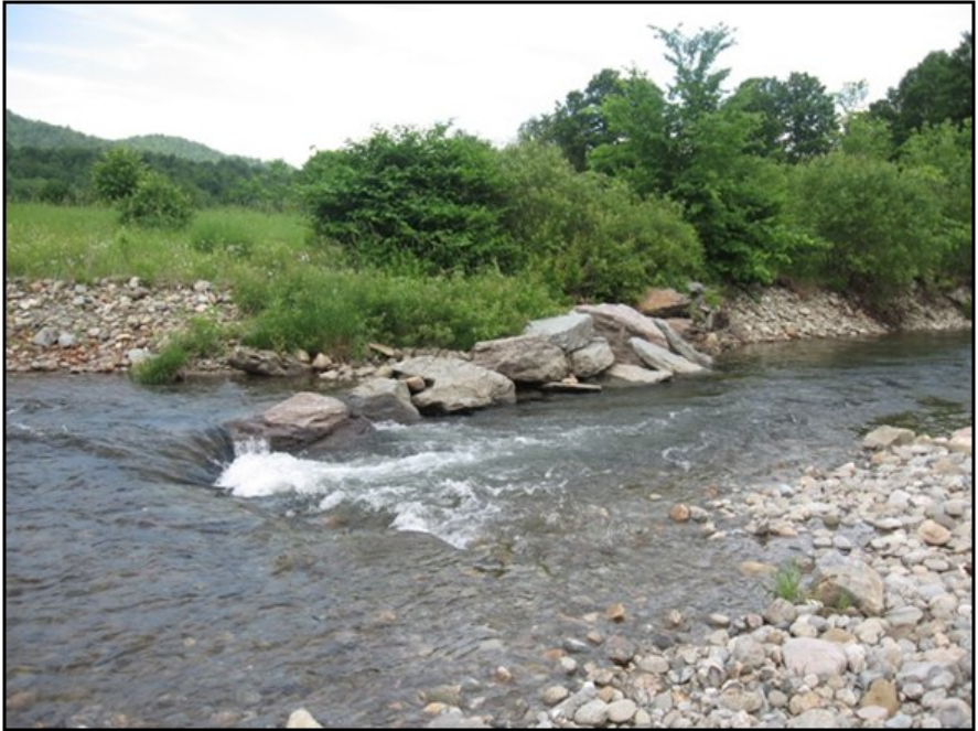
Figure 6. J-hook vanes meet multiple objectives including bank protection, sediment transport, channel capacity and habitat maintenance by dissipating and redirecting erosive energy into the center of the channel where a deep pool is created.
