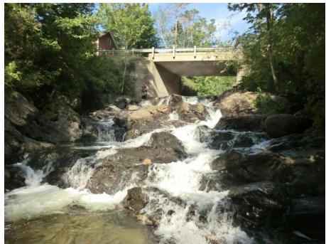
Example of ledge falls. A permanent grade control
