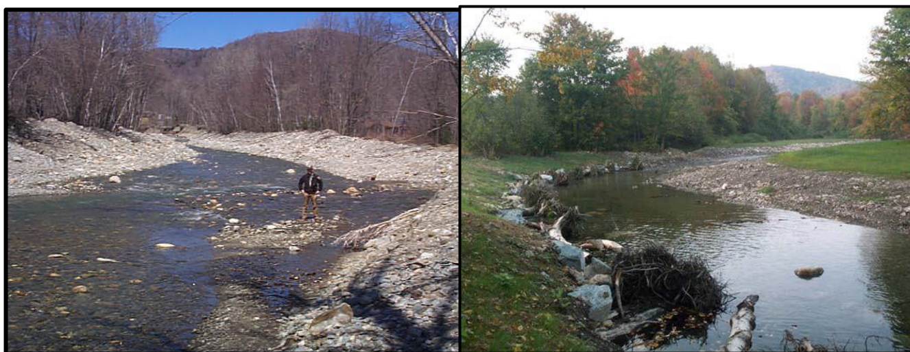
Before and after channel restoration on the White River in Granville, Vermont
