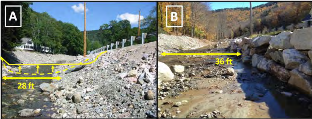
Figure 5.3-1: (A) Straigtened and windrowed channel on Pinney Hollow Brook along VT Route 100-A in Plymouth, Vermont following Tropical Storm Irene. (Source: Milone & MacBroom, Inc., September, 2011) (B) Completed placed riprap wall and natural stabilization of bed to increase bankfull width and cross-sectional area. (Source: Fitzgerald Environmental, October, 2013)
