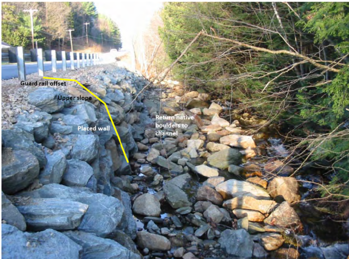
Figure 5.2-1: Placed riprap wall on the North Branch of the Hoosic River along Route 100 in Stamford, Vermont installed following Tropical Storm Irene where the roadway embankment and surface were eroded. (Source: Milone & MacBroom, Inc., 11/8/2012)
