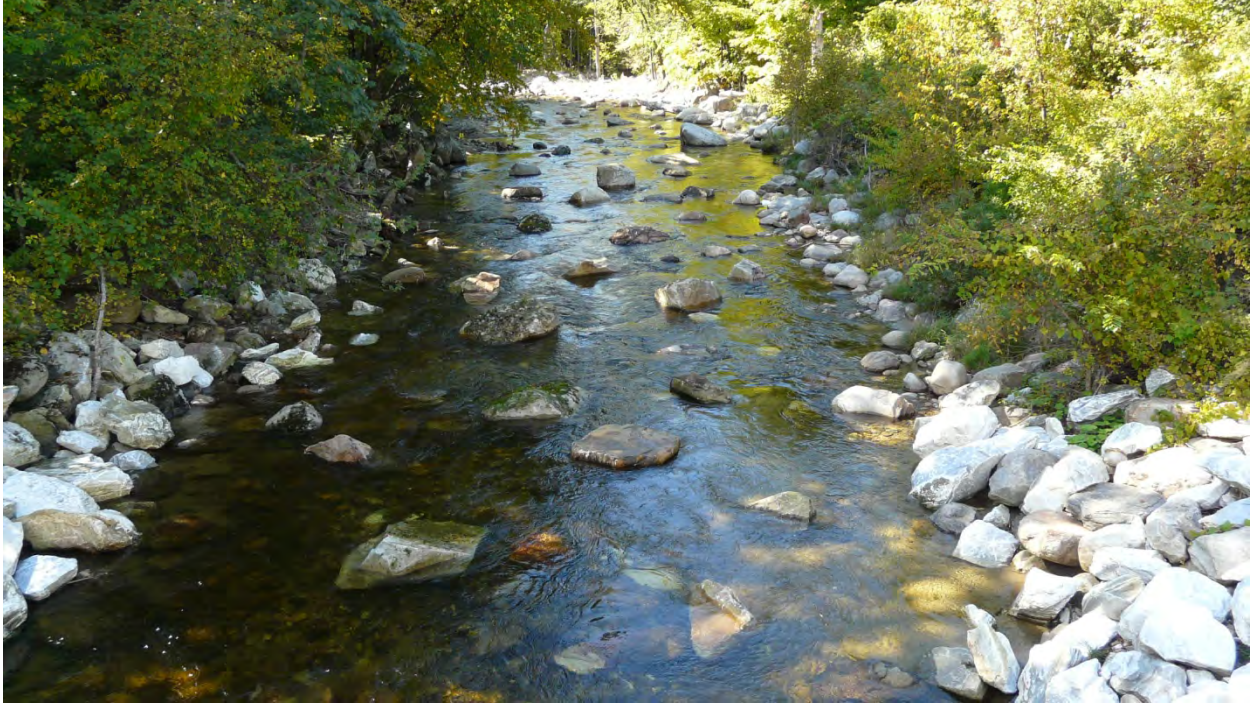
Figure 5.7-5: Roughened channel bed on the Middlebury River following boulder installation completed after sediment removal. (Source: Landslide Natural Resources Planning, 10/10/2013)
