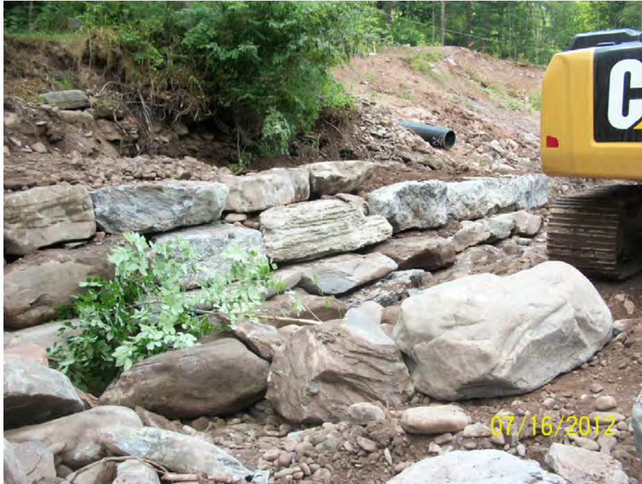
Figure 5.2-5: Stacked stone wall under construction on Stony Clove Creek in the Catskill Mountains, Chichester, New York. (Source: Milone & MacBroom, Inc., 7/16/2012)
