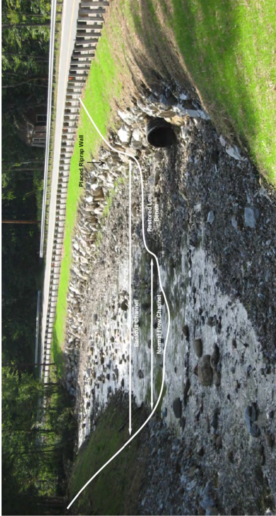
Figure 5.5-6: Photograph of restored low bench in conjunction with a placed riprap wall. (Source: Milone & MacBroom, Inc.). In a natural setting, the bench would form on the inside of the meander bend such as that associated with a point bar on a riffle-pool channel. The bench was left on the outside bend for this road protection project to properly narrow the channel to the reference bankfull width and reduce the channel work by leaving the work platform of native sediment in place. Migration of the channel thalweg toward the outside of the bend is anticipated over time.
