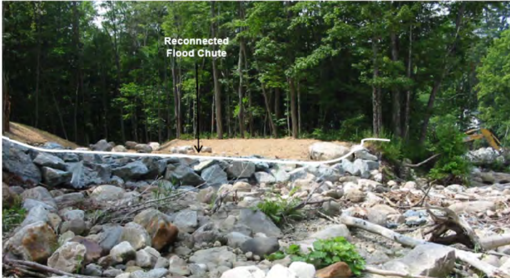
Figure 5.5-3: Reconnected flood chute on the Middlebury River in Ripton, Vermont to divert high floodwaters away from property and infrastructure. (Source: Milone & MacBroom, Inc. 2010)
