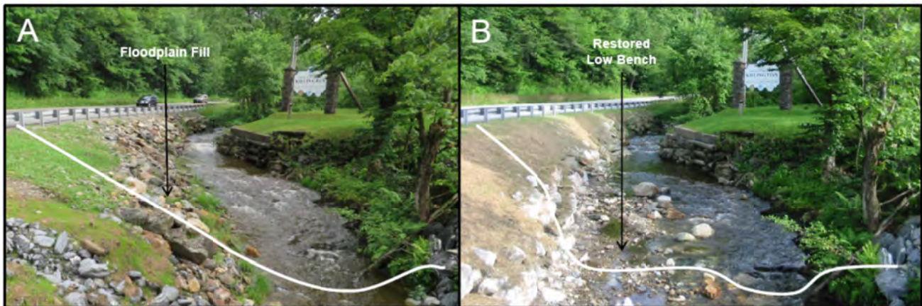
Figure 5.5-2: (A) Photograph of floodplain fill following emergency bank stabilization and road repair along the Tweed River in Killington, Vermont. (B) Photograph of the restored low bench after removal of the post-flood fill following permanent repairs. (Source: Milone & MacBroom, Inc., 2012)
