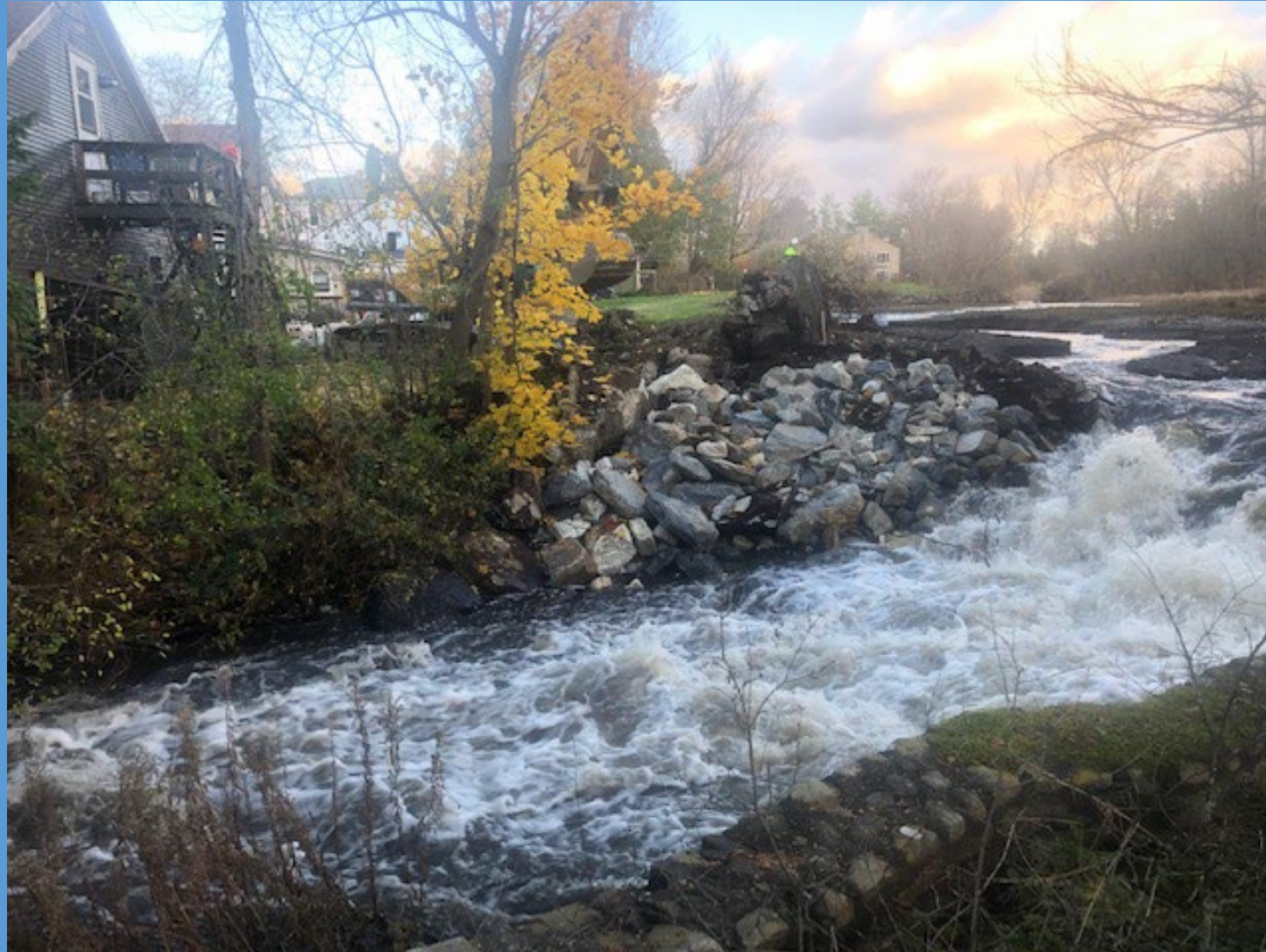
Looking Upstream at 2019 Partial Breach
