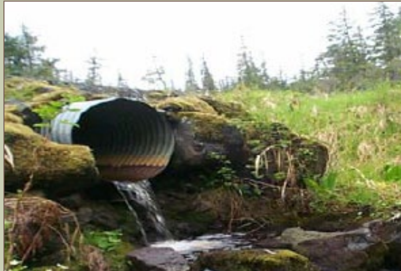
Culvert is a barrier
