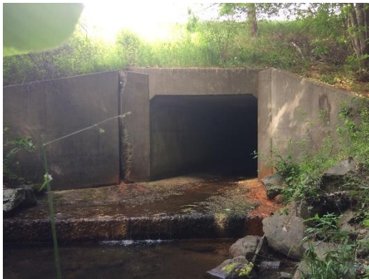
Figure 26. Example of a V bottom box culvert , with “dry concrete” movement surfaces along culvert walls. Site I91-17-2, Putney.
