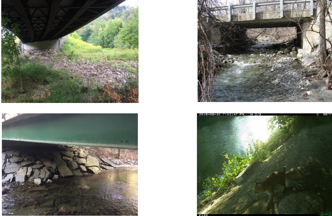
Figure 22. Examples of the variety of movement surface types that spans can provide. Upper left: “even floodplain” under valley-spanning bridge (9-25b, Searsburg). Upper right: “dry streambed” in a span with footing shelf where nearly all through-passages occurred on the streambed, which was typically entirely dry during summer months. Lower left: “riprap” streambank movement surface commonly found under many spans (not a project site). Lower right: “even streambank” of fine sediments under a span that does not cross an entire river valley (Union Street, Brandon, VT).
